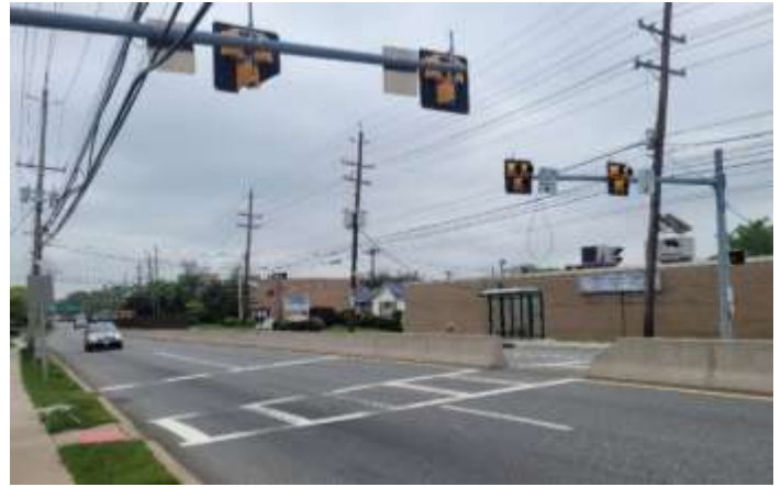
Pedestrian Hybrid Beacon (PHB) on Washington Avenue (County Route 503) in Carlstadt
